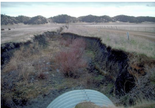
Gulley created by culvert in Bear Valley
